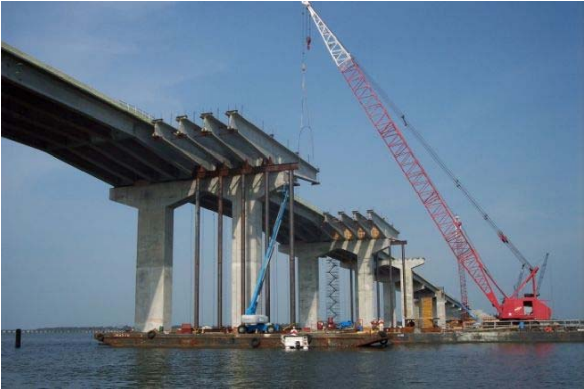
Figure 3 This is the U.S. 90 Bay St. Louis Bridge Located between Pass Christian and Bay St Louis, MS
